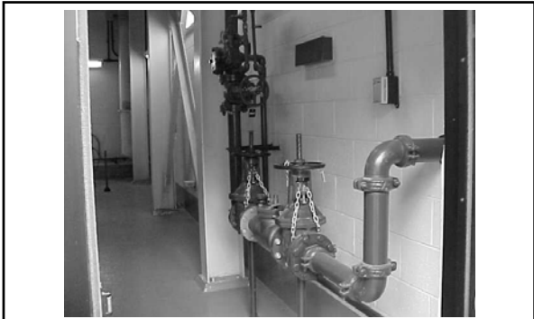
Sprinkler System in Chlorine Room ?
