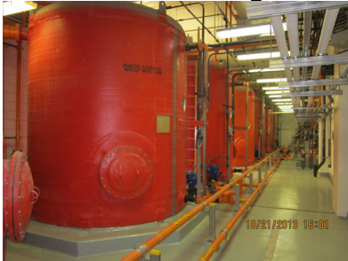
FRP Bulk Storage
