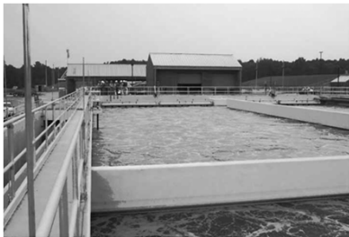
Aeration of BNR/ENR Processes
