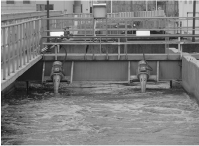
Aeration of BNR/ENR Processes
