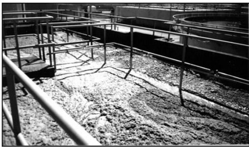
Nocardia Foam on the Surface of Aeration Basin
