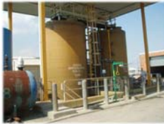
Sodium hypochlorite tanks
