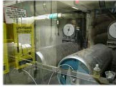
1-ton chlorine cylinders
