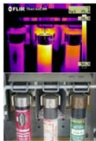
Fuses Hot fuse connection.
