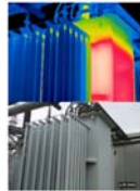
Transformer Cold cooling fins due to low oil level in a transformer.
