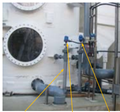
Element of filling tube (type) Sump High level switch Sump Level Transmitter (LRT)
