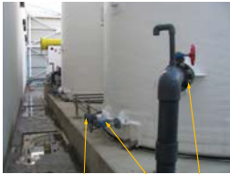
Sump heating element Temperature Indicating Transmitter Sump high level overflow
