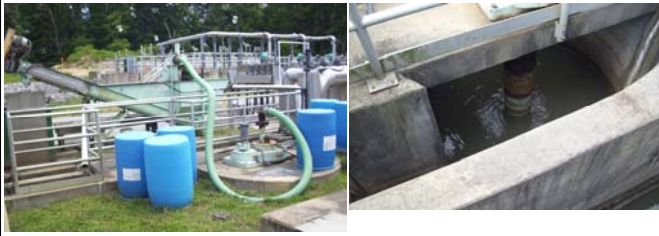
Grit Removal – Pista Grit w/ air lift
