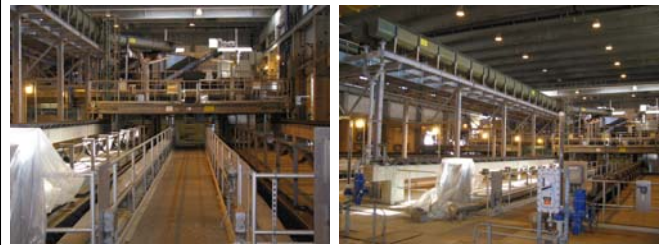
Grit Removal – Traveling Bridge
