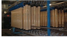
Microfiltration water plant, Petrolia, PA
